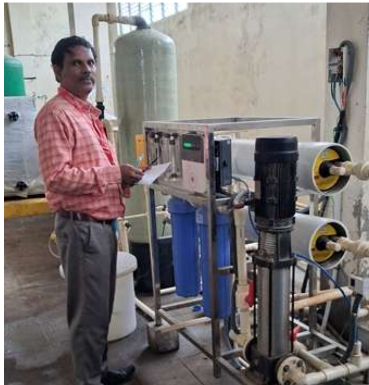
KBA MEN'S HOSTEL RO PLANT
