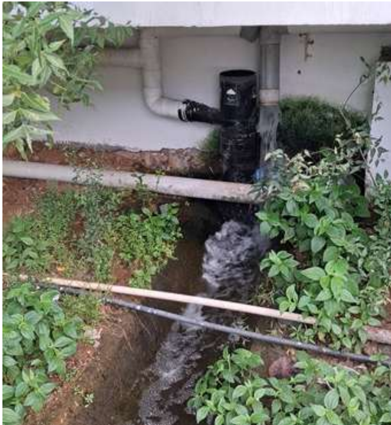
Water over Flow
